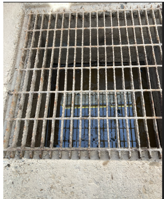
Example of sump with solution
