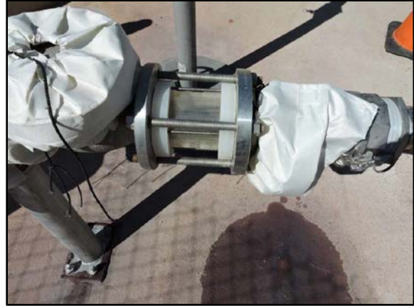
Figure 5.1 Improper installation of flange cover leading to damaged flange cover (diaper)
