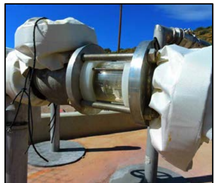
Sight Glass and Flange Covers (Diapers)
