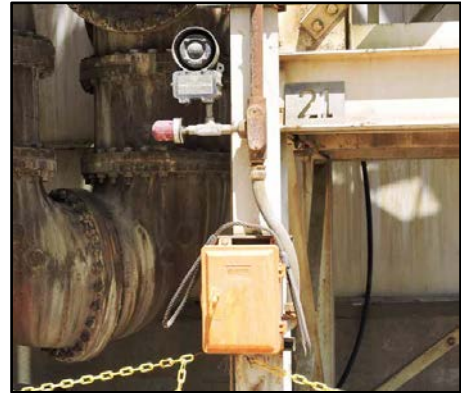
Figure 3.2 GAI-Tronics Intercom and Handset
