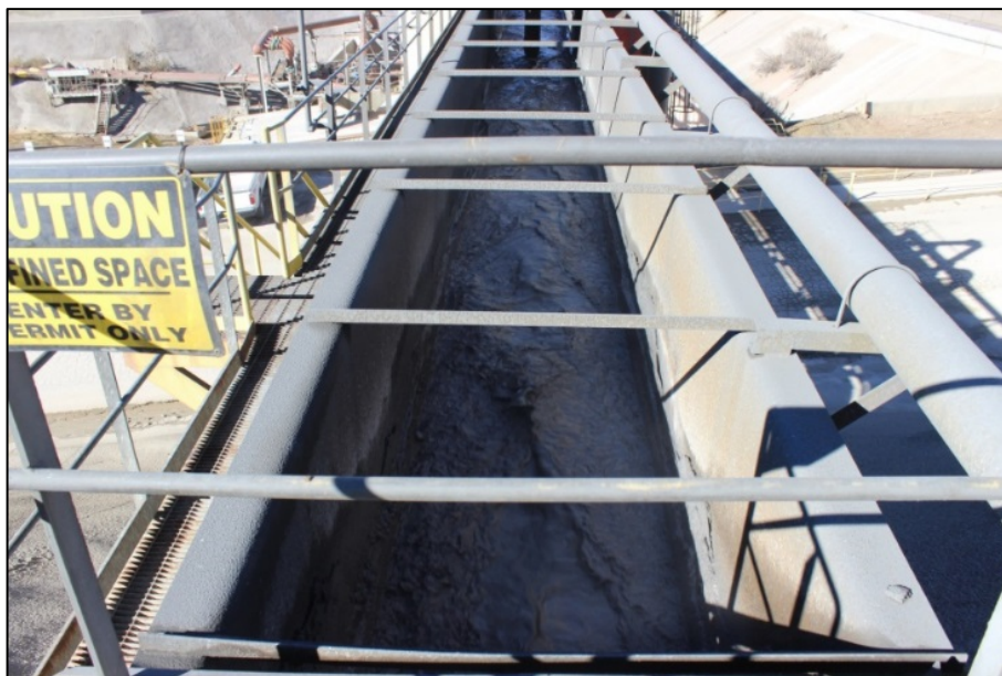
Fig. 4 Tail launders have limited entry and exit locations
