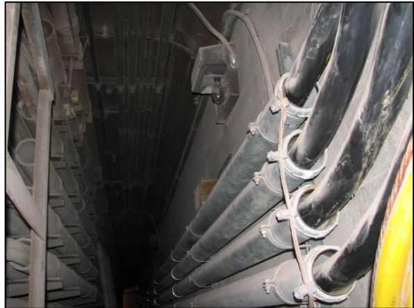
Fig. 23 Electrical conductors under a concentrator
