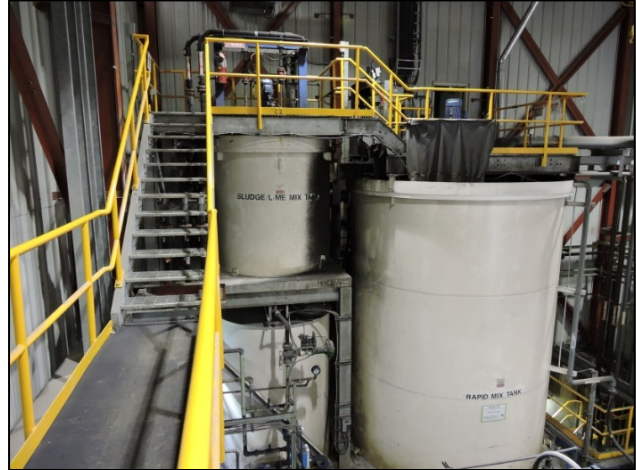
Fig. 24 Mechanical hazards exist inside tanks
