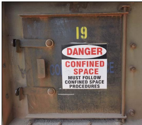
Fig. 31 Signage on a chute entrance is an administrative control
