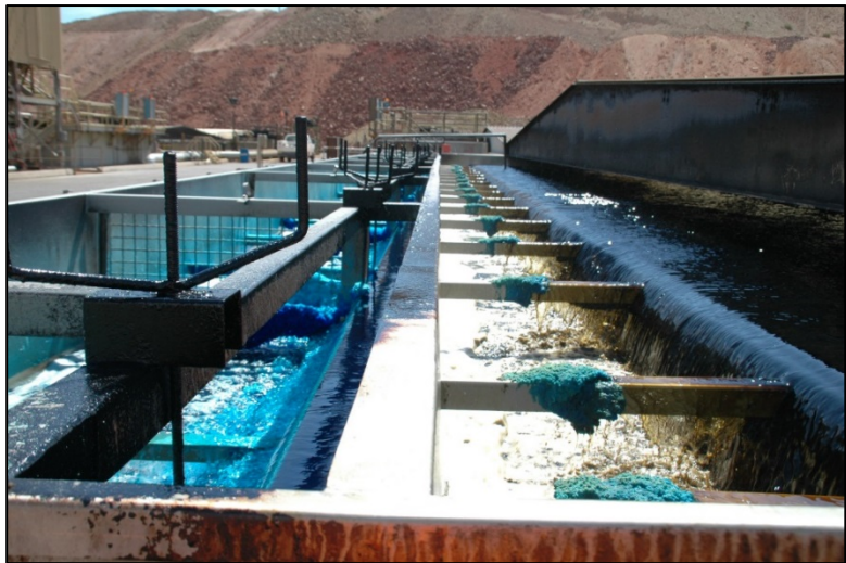
Fig. 9 Chemical hazards at SX settlers
