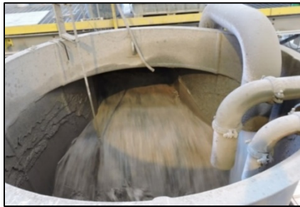
Fig. 7 Tank has the potential for engulfment
