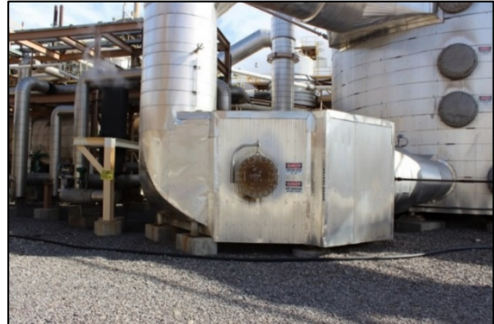
Fig. 11 Acid plant has atmospheric hazards
