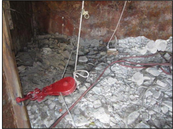
Fig. 28 Be Aware of Tripping Hazards
