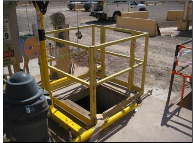
Fig. 50 Temporary guarding protecting an opening
