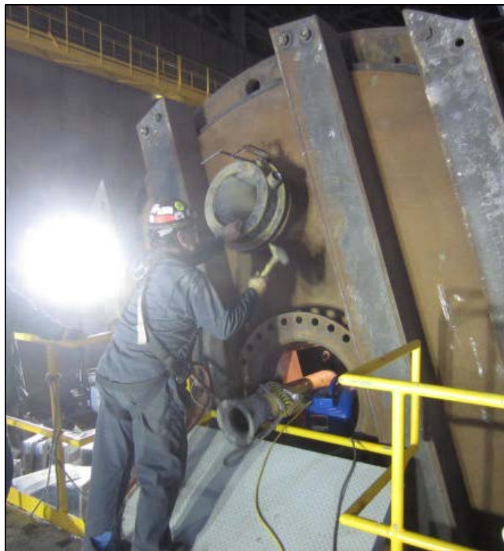
Fig. 51 Lighting is used to illuminate this confined space
