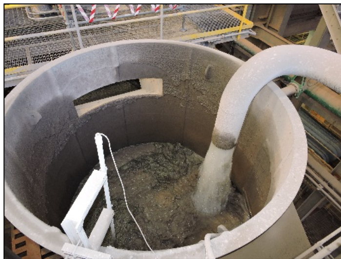
Fig. 21 Potential for engulfment in this tank
