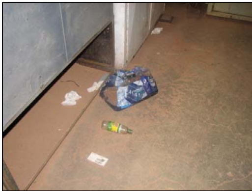
Fig. 15 Trash and debris
