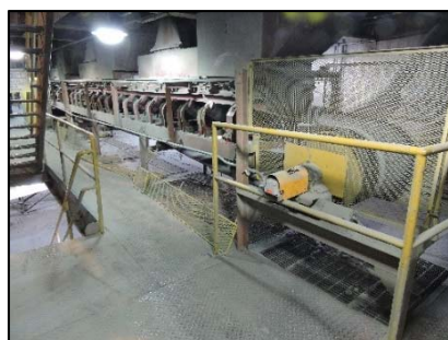
Fig. 12 Guarding left on the ground
