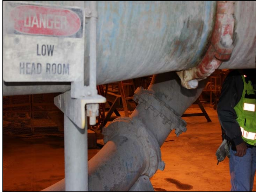
Existing Hazard(s) / Potential Consequence
