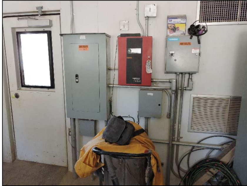
Existing Hazard(s) / Potential Consequence
