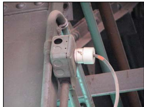
Fig. 21 Missing knockout plug
