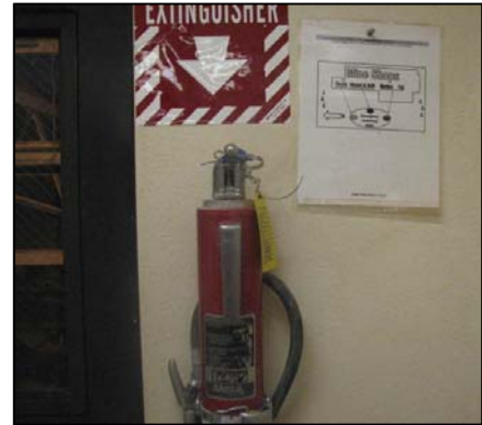
Fig. 28 Fire extinguisher in the workplace
