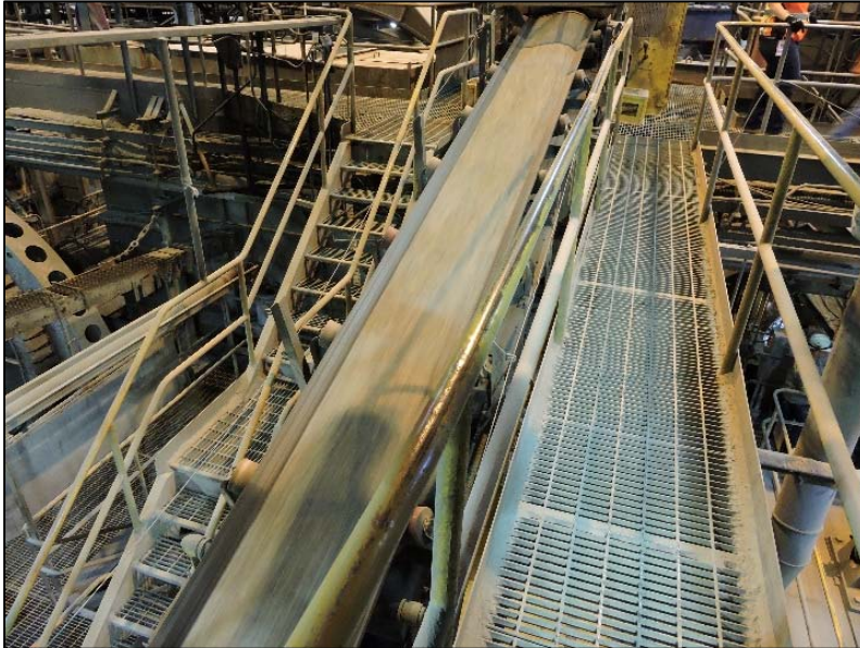
Fig. 36 Walkway and stairs along a conveyor
