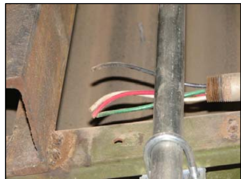
Fig. 22 Exposed wiring on a conduit
