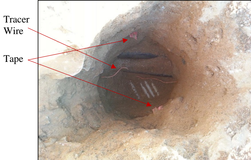
Figure 3.1 Tracer wire and tape indicating nearby utility pipes/conduit
