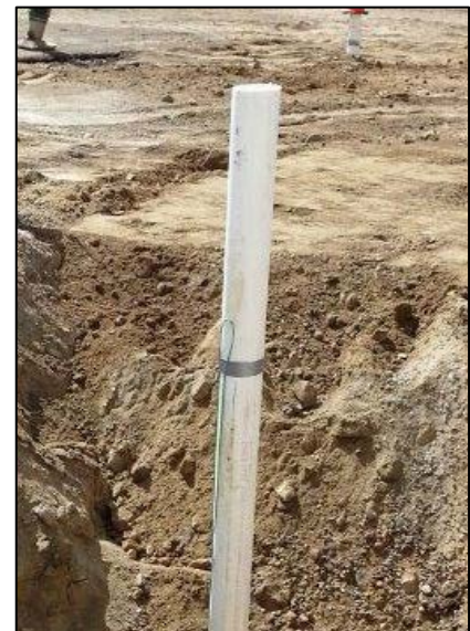
Figure 3.3 Tracer wire seen taped to conduit above the ground level
