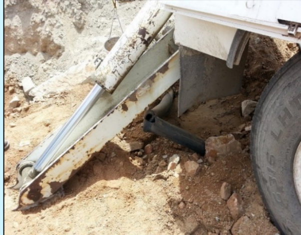
Figure 1.3 Improper placement of a crane
