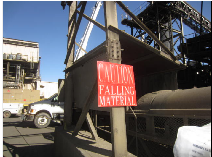
Fig. 2.5 Warning sign permanently installed
