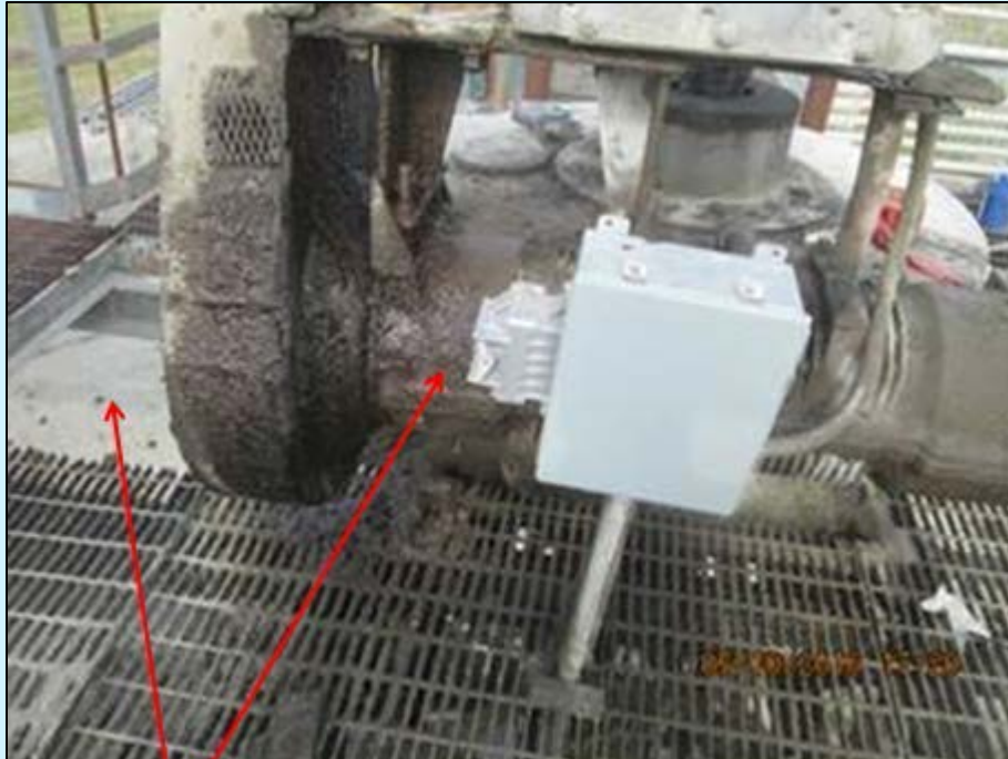
Fig. 2.12 Arrows indicate missing grating (left) and control switch for his task (right)
