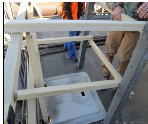
Fig. 10 Handrails around the hatch
