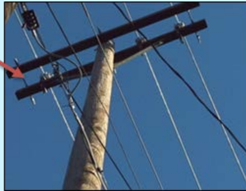
Fig. 23 Where employee wanted to tie off
