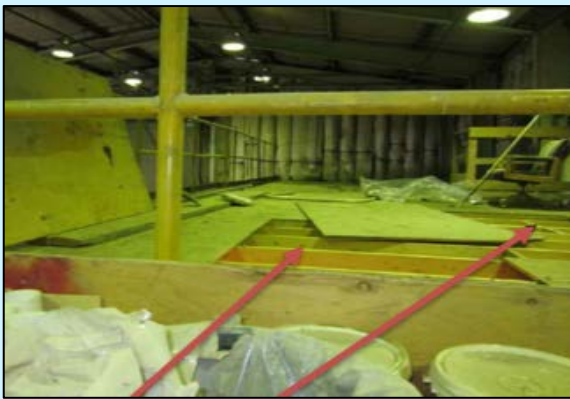
Fig. 1 Mezzanine floor where plywood was removed above false ceiling
