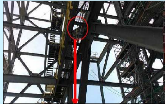
Fig. 16 Gap between floor grating sections
