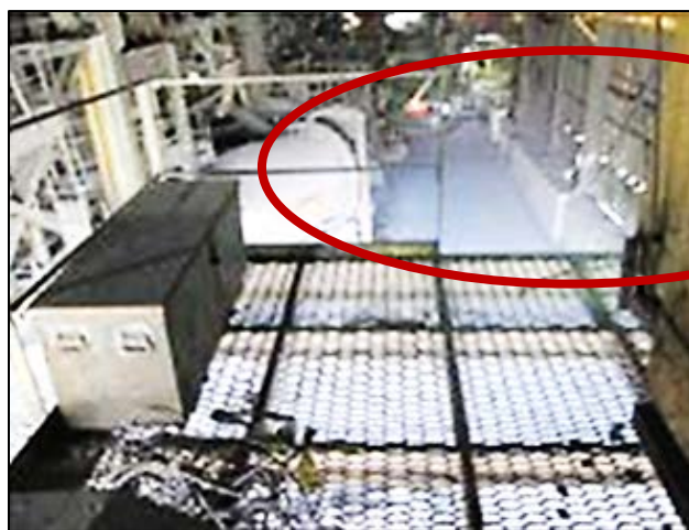
Fig. 5 Crane bay platform with missing gate
