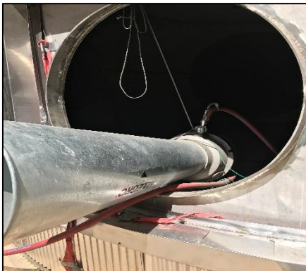
Figure. 2.2 Local exhaust ventilation being utilized.
