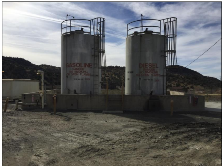
Figure 7.1 Fuel storage at the Tyrone Mine Site.
