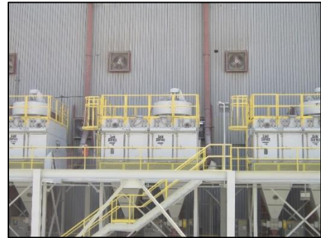
Figure 7.6 High Hazard Area- FARR Unit Dust Collection System
