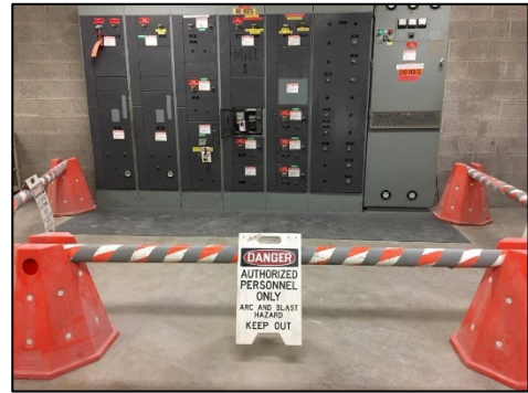
Fig. 2.25: MCC bucket racked out and locked out (electrically safe), with flagging and barricading
