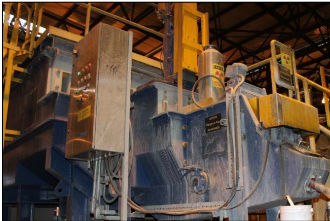
Fig. 1.14 On-Stream Analyzer (OSA)
