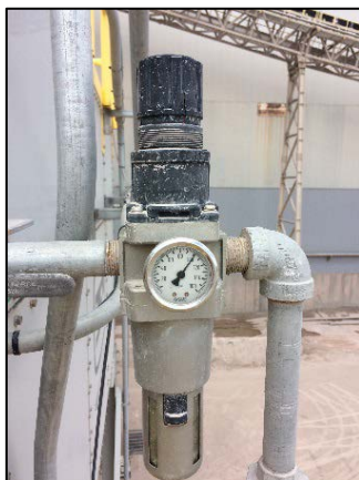
Fig. 1.16: Stationary compressed airline
