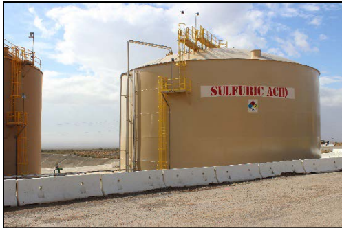
Fig. 1.5: Sulfuric Acid tank
