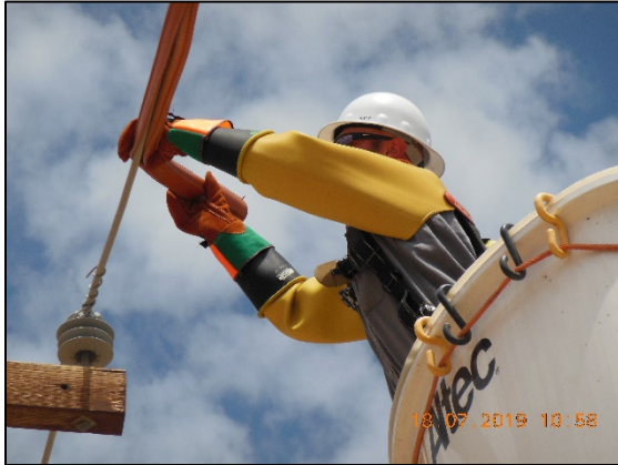
Fig. 2.29: Insulating blanket over power line
