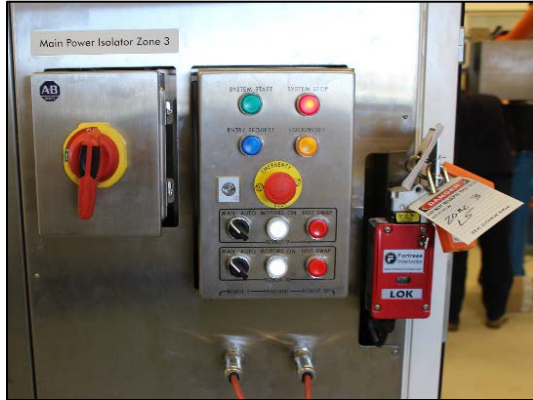
Fig. 2.16: Control panel for an electrical device
