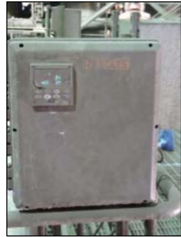
Fig. 2.34: Labeling difficult to read
