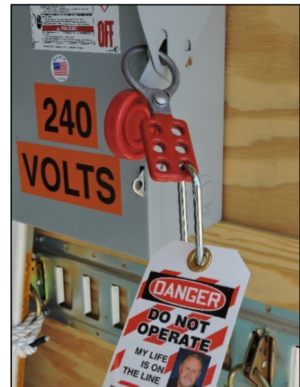
Fig. 2.15: Simple lockout on a switch
