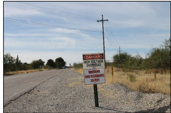
Fig. 1.4: Overhead power lines
