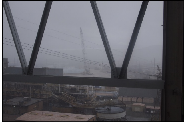
Fig. 3.18 Rainy weather creates new hazards.
