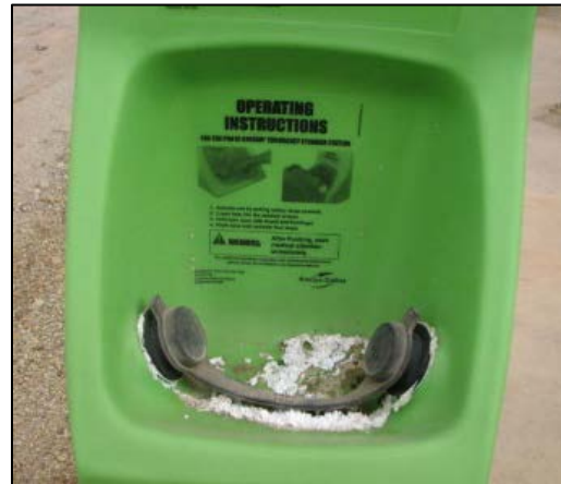
Fig. 3.25 Eyewash station with build-up.
