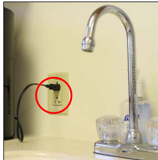
Fig. 3.12 GFCI on an outlet near a sink.
