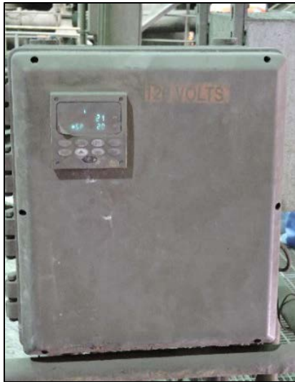
Fig. 3.13 Labeling that is difficult to read.
