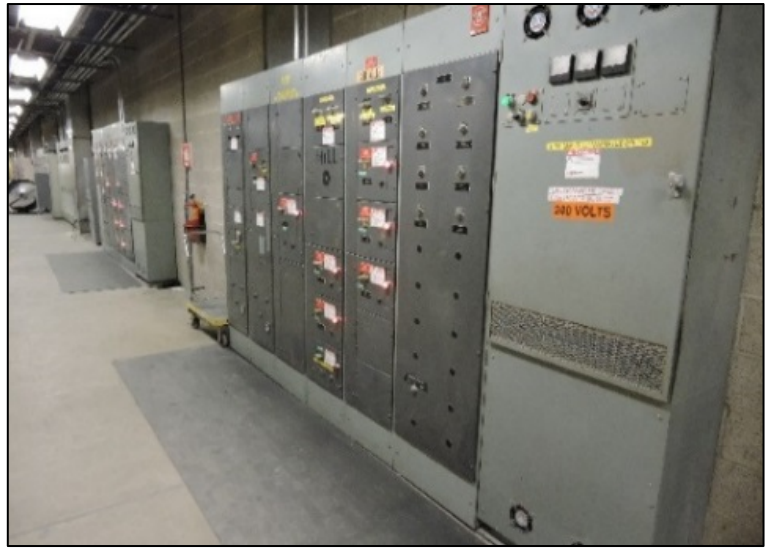
Fig. 3.7 Electrical panels in a work area.
