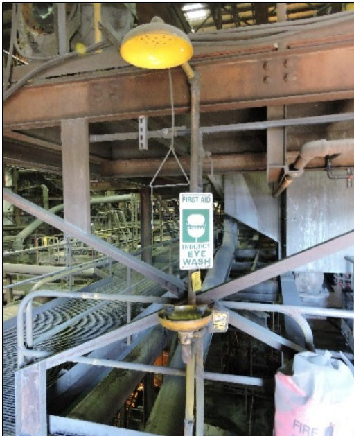
Fig. 3.24 Eyewash station and shower.
