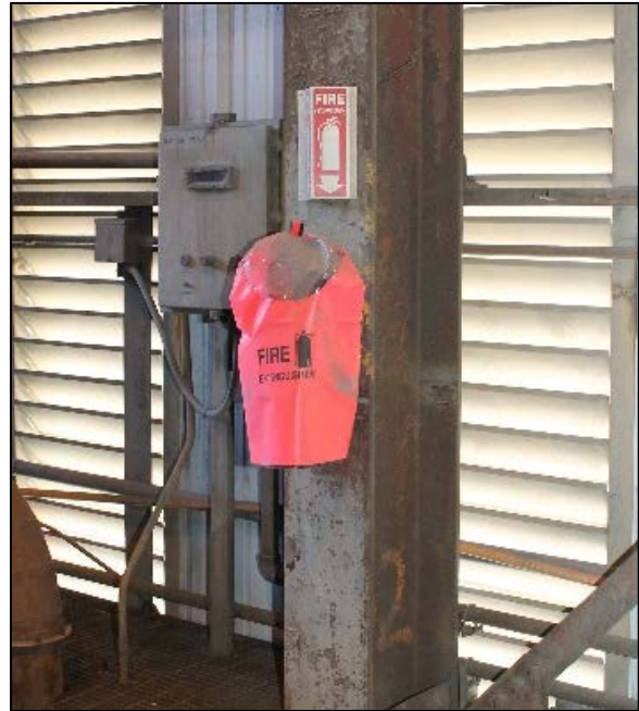
Fig. 3.26 Fire extinguisher in the workplace.
