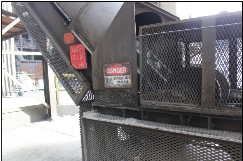
Fig. 3.4 Proper guarding protects employees from moving parts.
