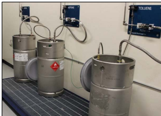
Fig. 3.33 Chemical containers with proper labeling.
