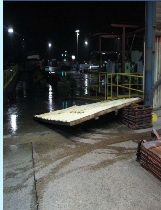
Fig. 2.6 Another angle of the fallen door.
