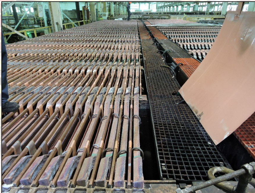
Fig. 1 A missing cathode creates a hazard. Remain aware of hazards as you work.
