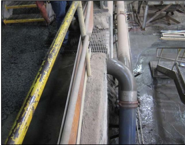
Fig. 3.20 Material spillage leads to slipping incidents.
