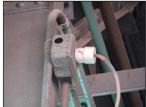
Fig. 2.3 Missing knockout plug
