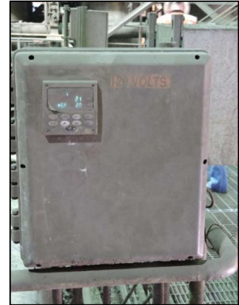
Fig. 2.5 Panel is difficult to read
