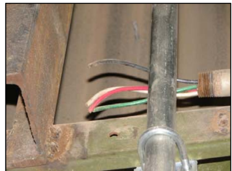
Fig. 2.4 Exposed wiring on a conduit
