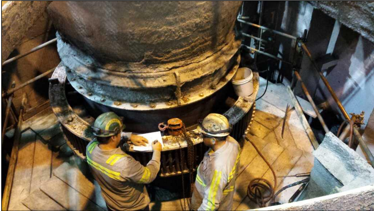
Figure 1.9: Employees evaluating new hazardous condition
