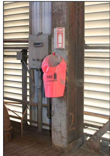
Figure 2.5: Fire extinguisher location
