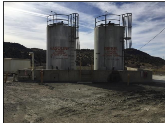
Figure 6.1: Fuel storage area
