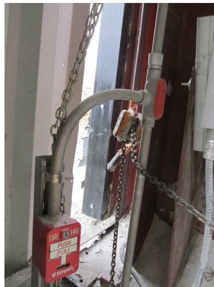
Figure 5.6: Poor rigging practices
