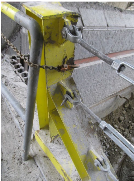
Figure 5.5: Poor rigging practices
