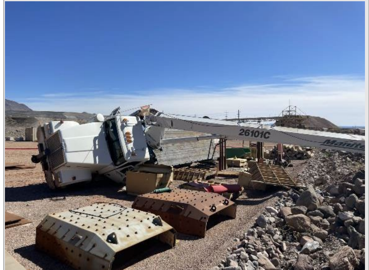
The boom truck tipped onto the driver's side when the load swung.
