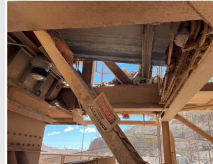
Spillage on edge of support beams over dribble chute on second level.
