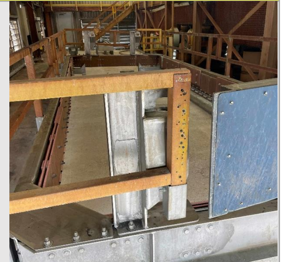
Area the operator's leg contacted the jumper frame
