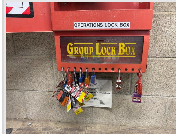
Operations lock box. Contractor was locked on this box without the ECC lock.
