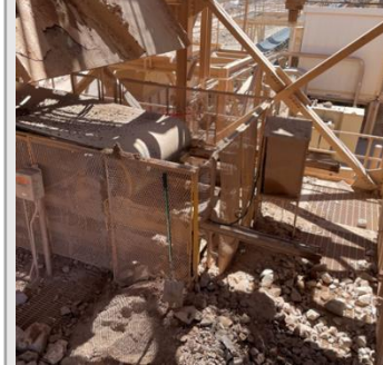
Area where rock fell.
