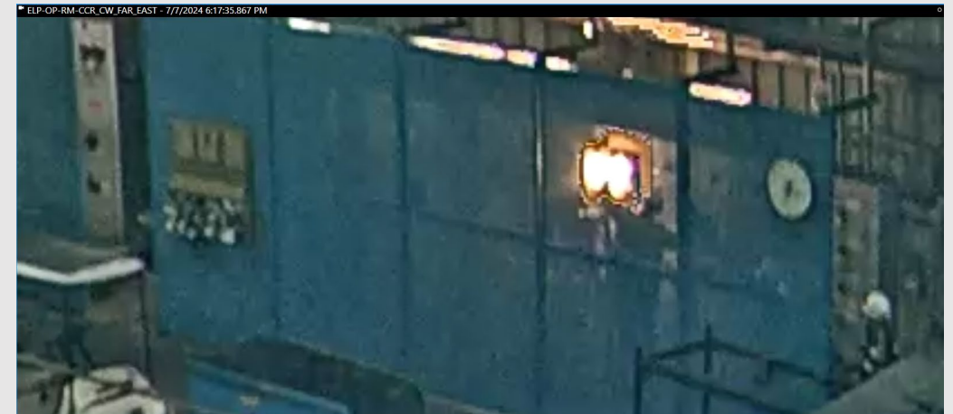
Electrician inside of the motor control center when arc flash occurred
