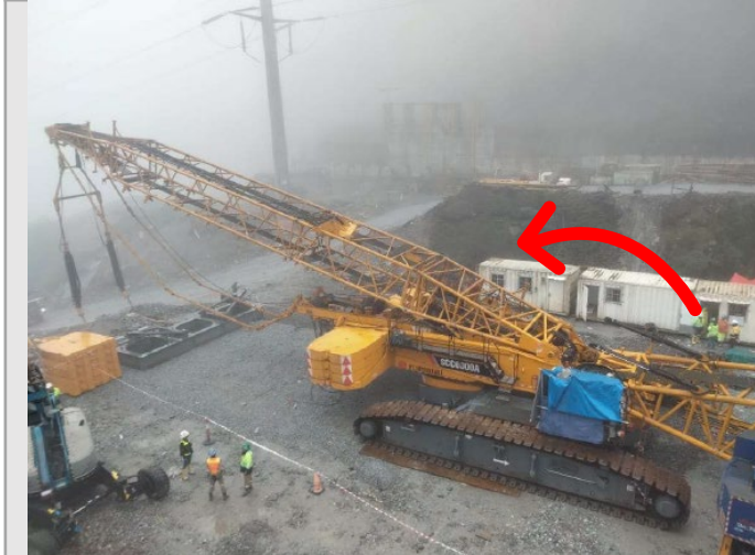
Super lift mast collapsed backward over car body.
