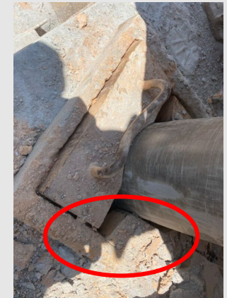
Top view where steel wedge was installed and later dislodged.
