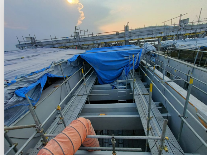
The scaffolding where the worker fell.
