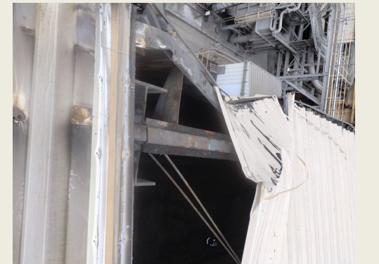
Damage to the roof
