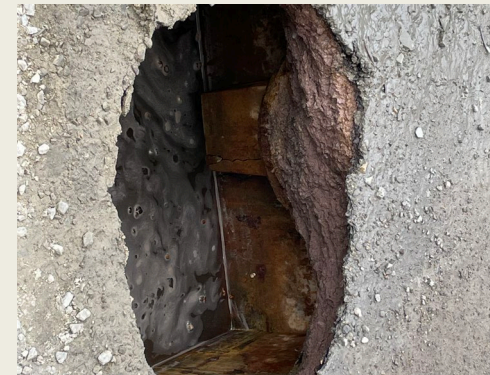
Cavity that the outrigger fell into
