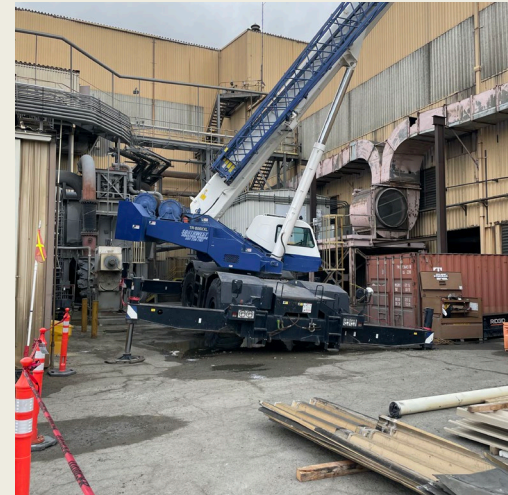
Position of the crane after the event
