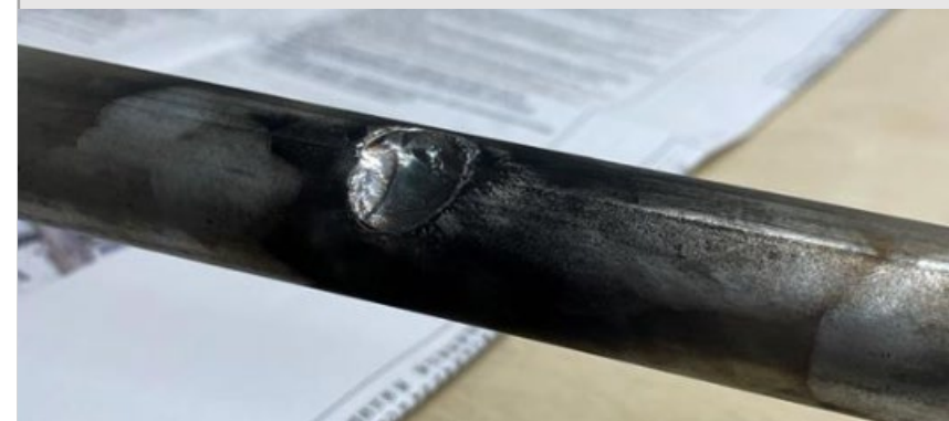
Conduit that contacted the 480v line
