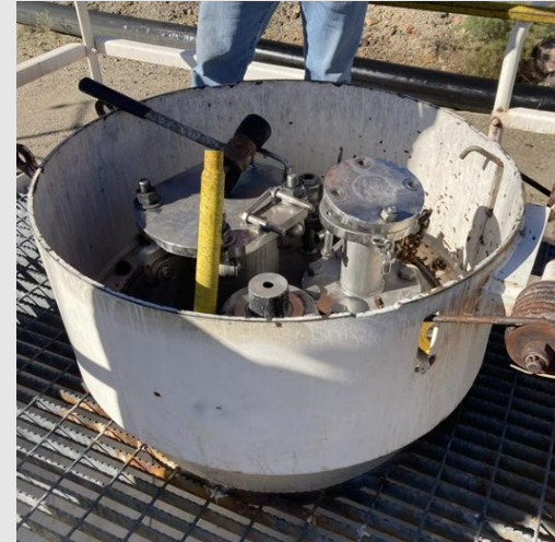
Flange where bolt was cut.
