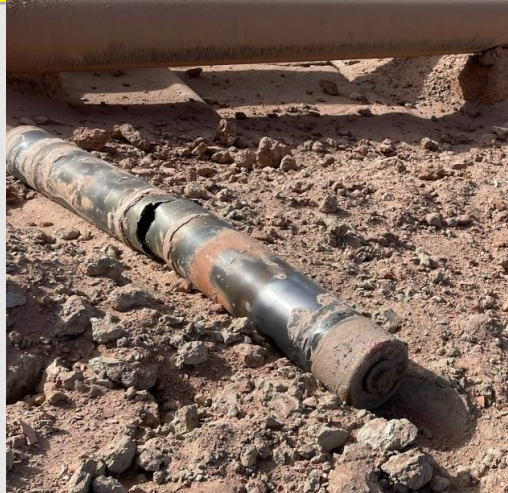
Worn idler that fell from conveyor
