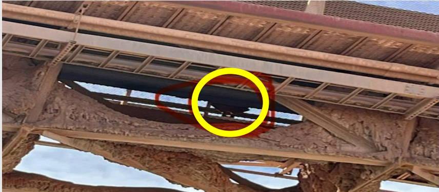
Idler fell from section of conveyor circled in yellow
