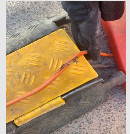
Failed extension cord.
