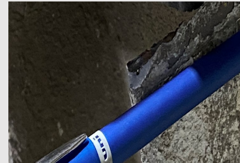
Mounting plate failure
