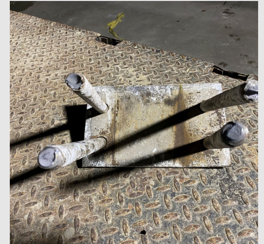
Sheared retaining bolts
