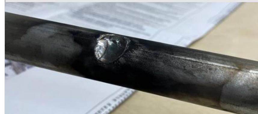
Conduit that contacted the 480v line
