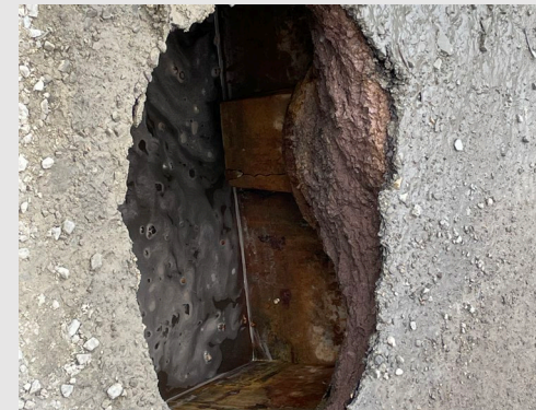
Cavity that the outrigger fell into
