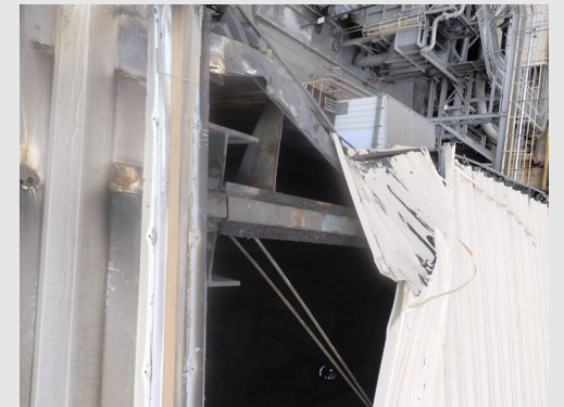
Damage to the roof
