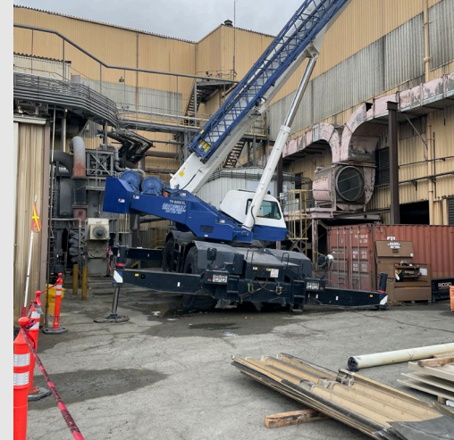
Position of the crane after the event
