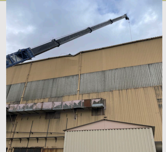
Location of where the crane hit the roof
