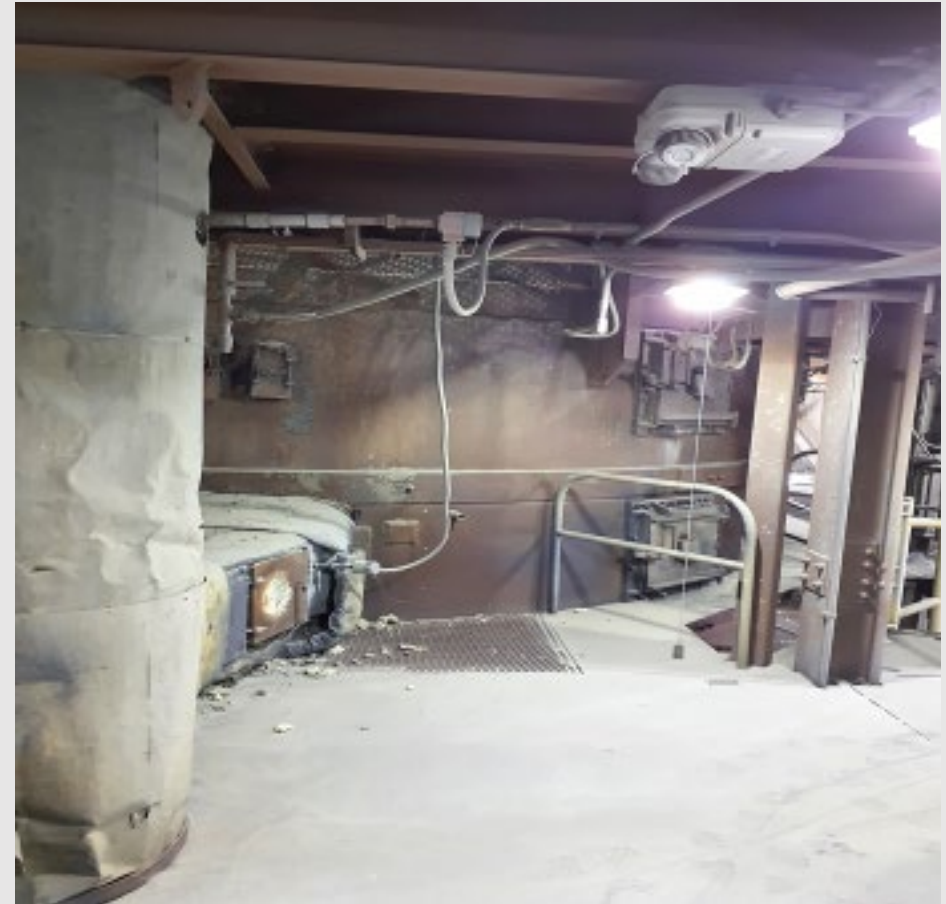
The building electricians entered and were exposed to sulfur dioxide gas.
