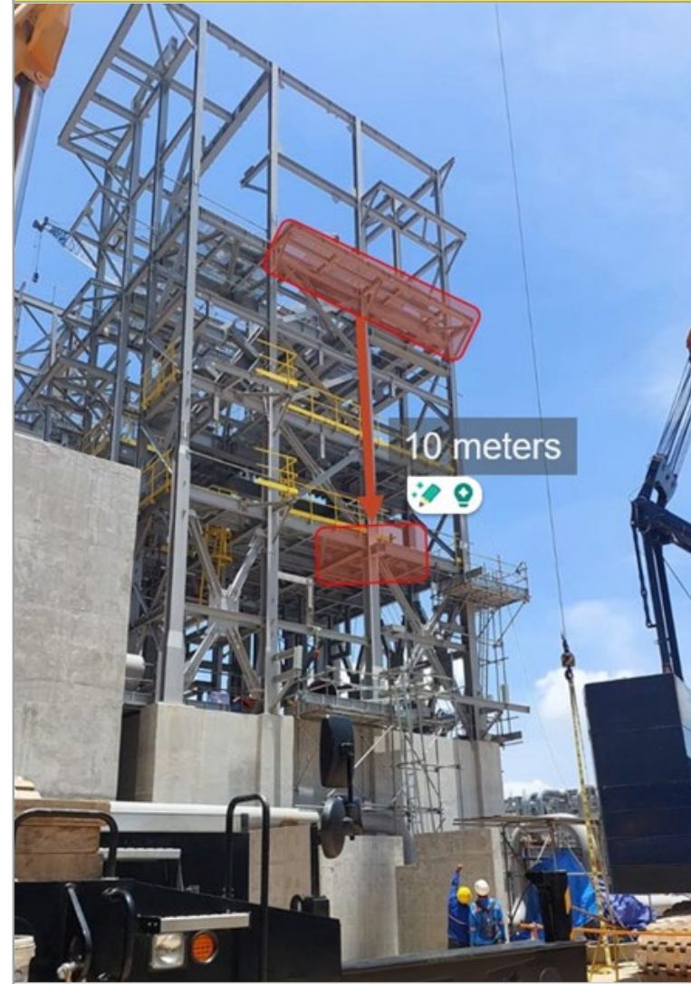
Scaffold grating weighing 20 kilograms fell 10 meters, striking an employee in a man basket.
