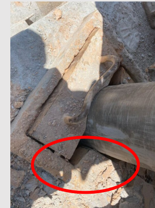
Top view where steel wedge was installed and later dislodged.
