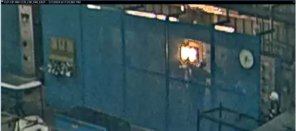
Electrician inside of the motor control center when arc flash occurred
