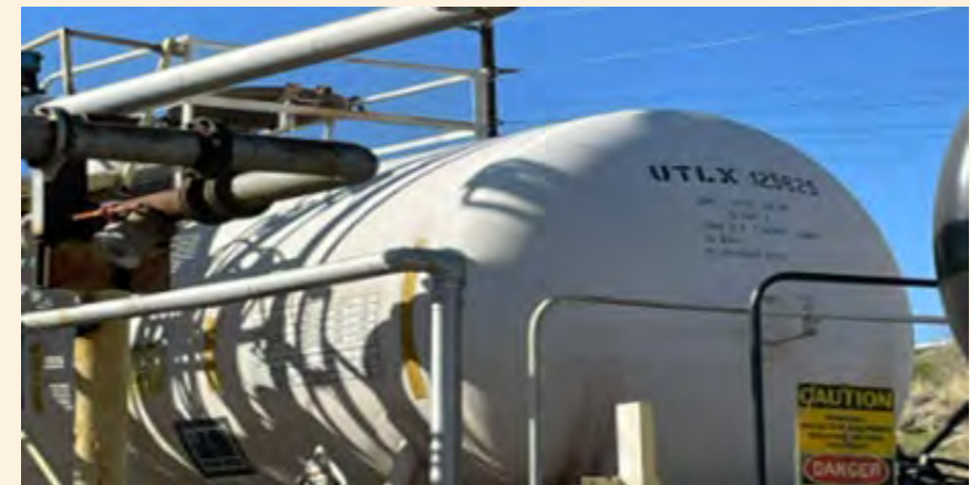
• Work platform above the acid tanker car.
