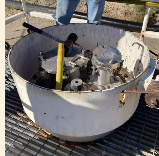
• Flange where bolt was cut.
