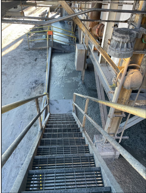
Sheer Feed containment area – one side yellow flagging/ bottom of stairs still accessible
