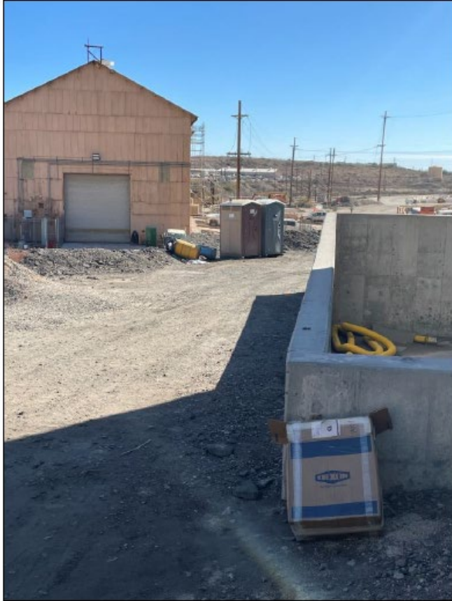
Full trash can /hand wash station tipped over/ Not cited
