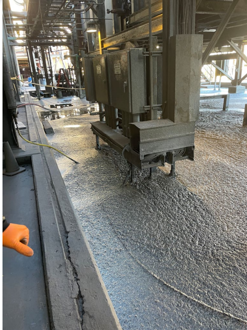
Sheer Feed containment area – one side yellow flagging/ open to all other sides
