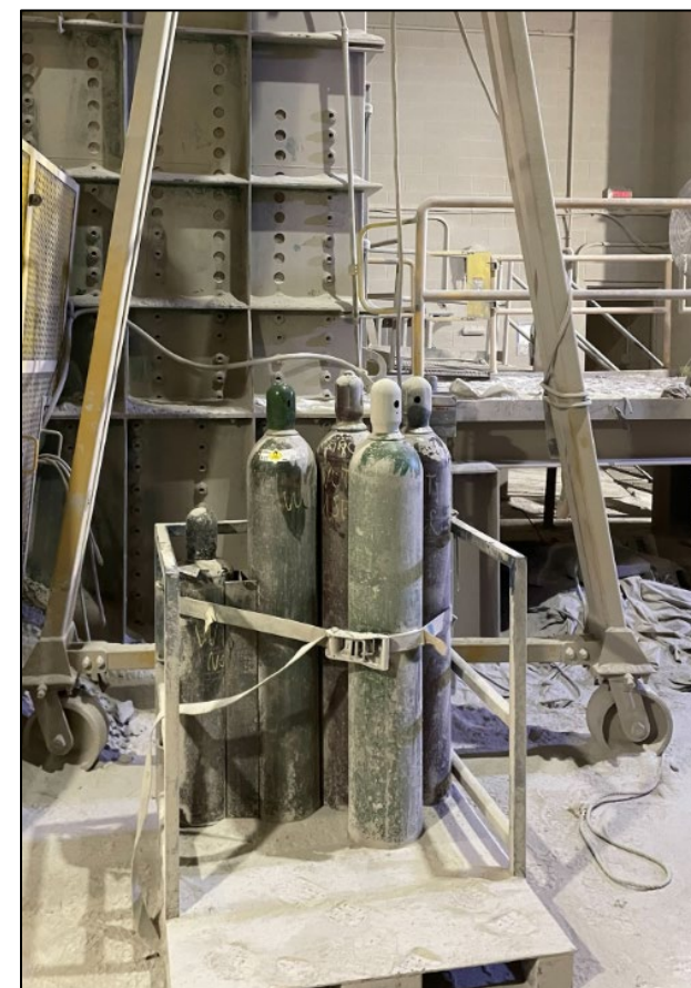
Gas cylinders stored at crusher 3 without no smoking/flames warning sign. 56.7805 Fire
