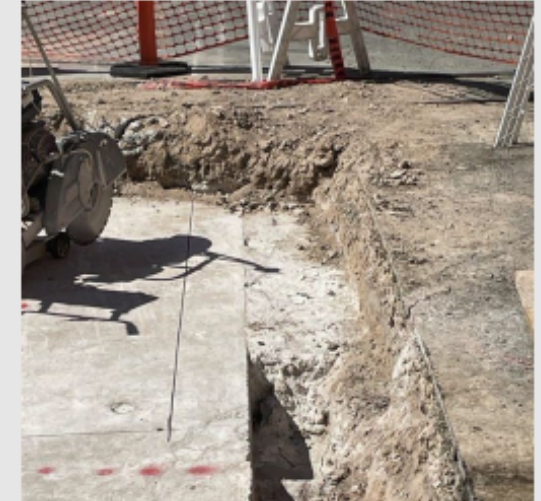
Excavation made outside of white paint
