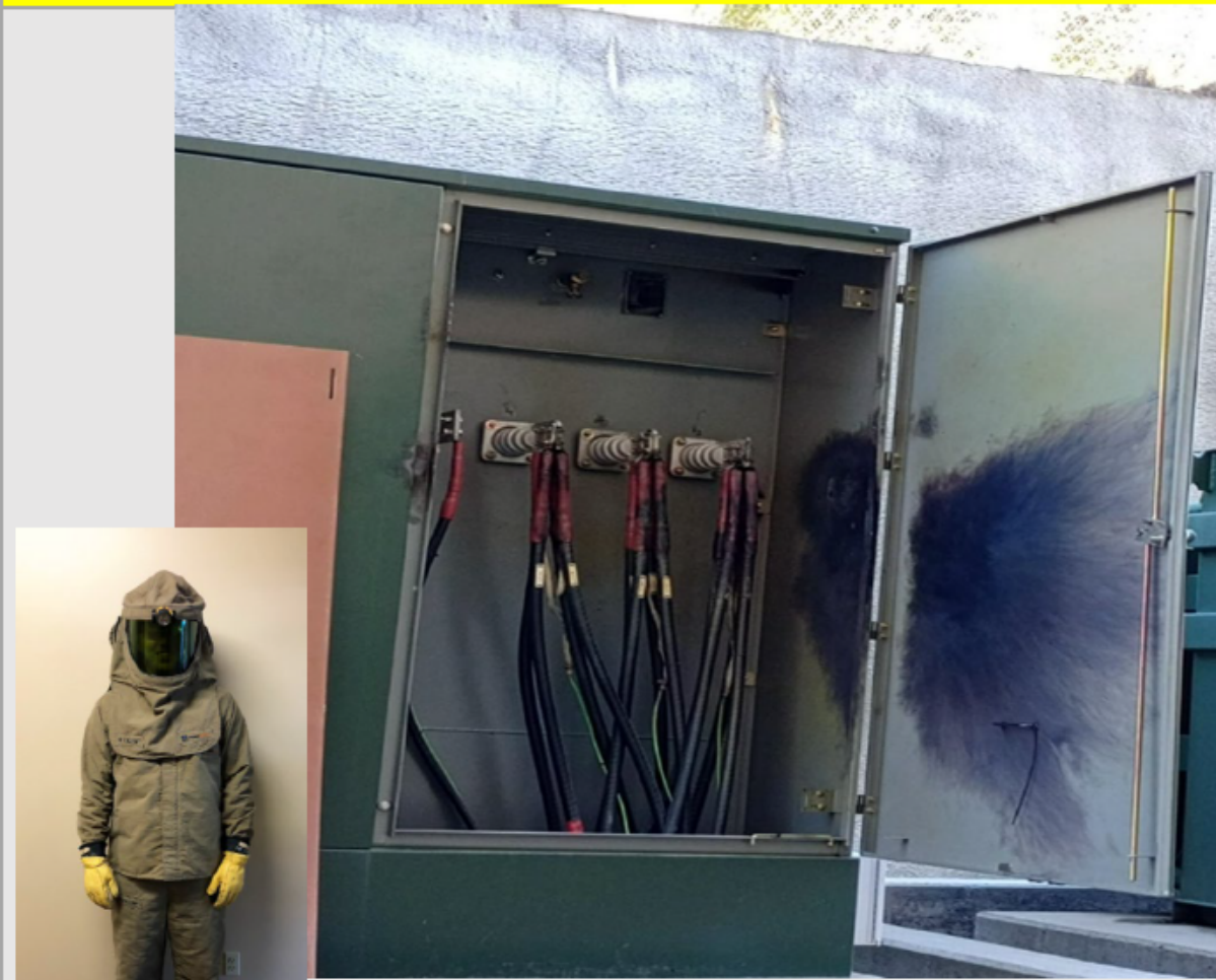
At left: Proper PPE required for the job (not worn during the incident)
