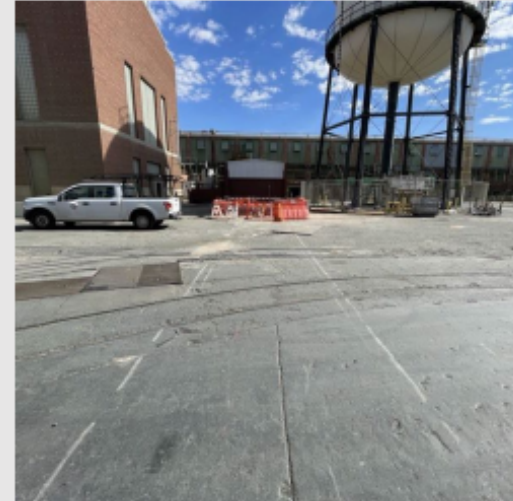
Area marked for excavation; not all utilities marked with correct color
