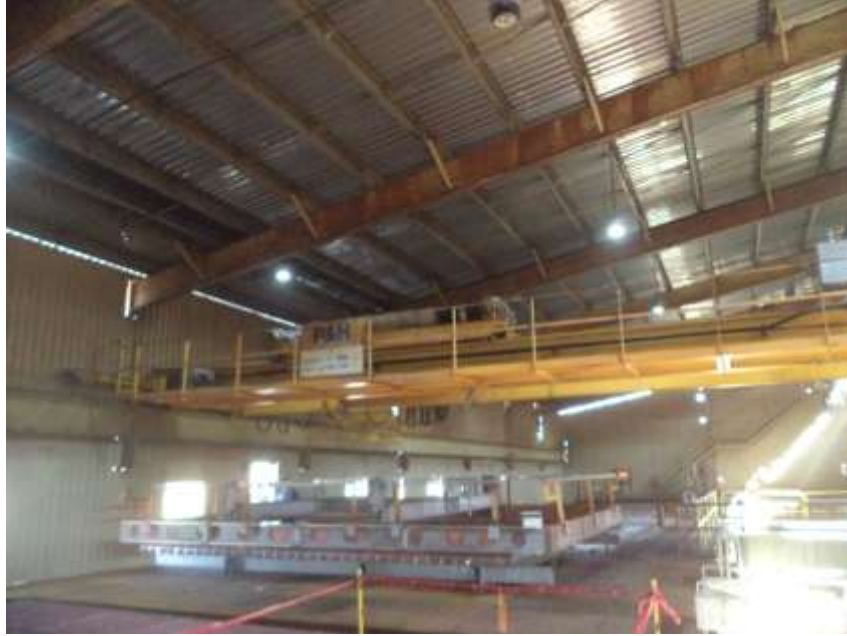
The load was approximately 4 feet off the cell line when the failure occurred
