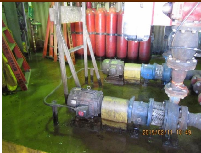
Flooded Caustic Building
