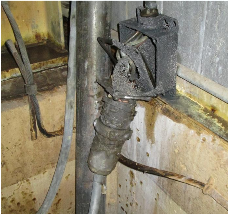
480V extension cord connection
