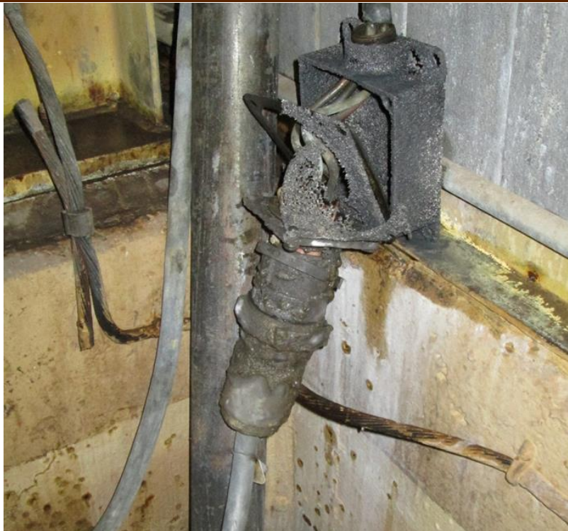
480V extension cord connection
