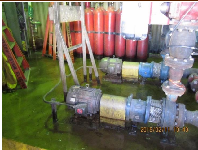
Flooded Caustic Building
