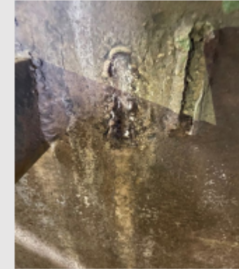
Broken guard welds
