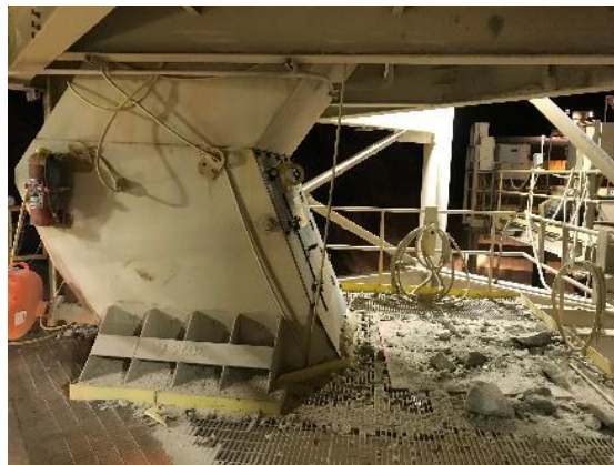
Photo 2 Chute being inspected. Chute contains a total of six air cannons, however it is uncertain which one fired first. An air cannon can be seen to left of photo.
