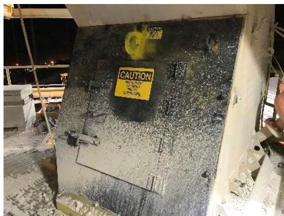
Photo 3 Inspection chute door with air cannon on right side.
