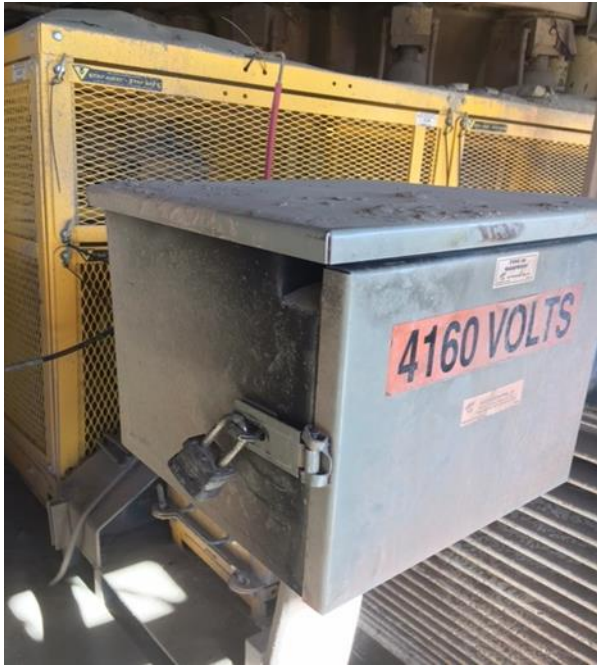
Motor tap box after arc flash
